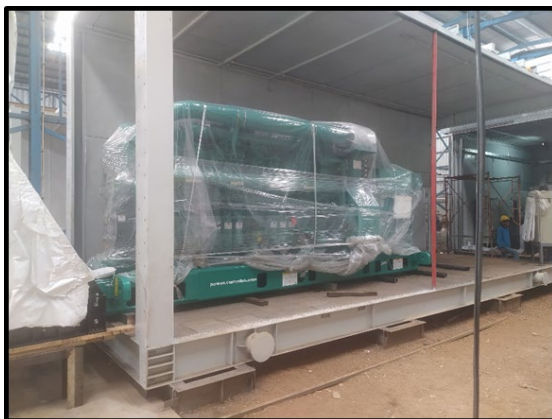
Gambar 4. Generator Cummins QSK 95 G4
